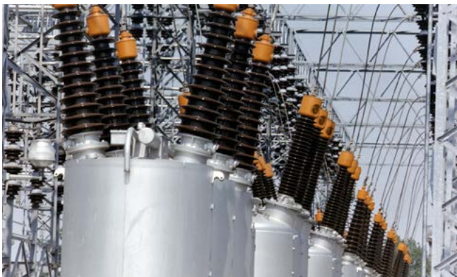
The U.S. electricity grid requires modernization to safely and reliably accommodate demand and integrate renewable energy sources and emerging technologies. (Energy.gov/Flickr)
